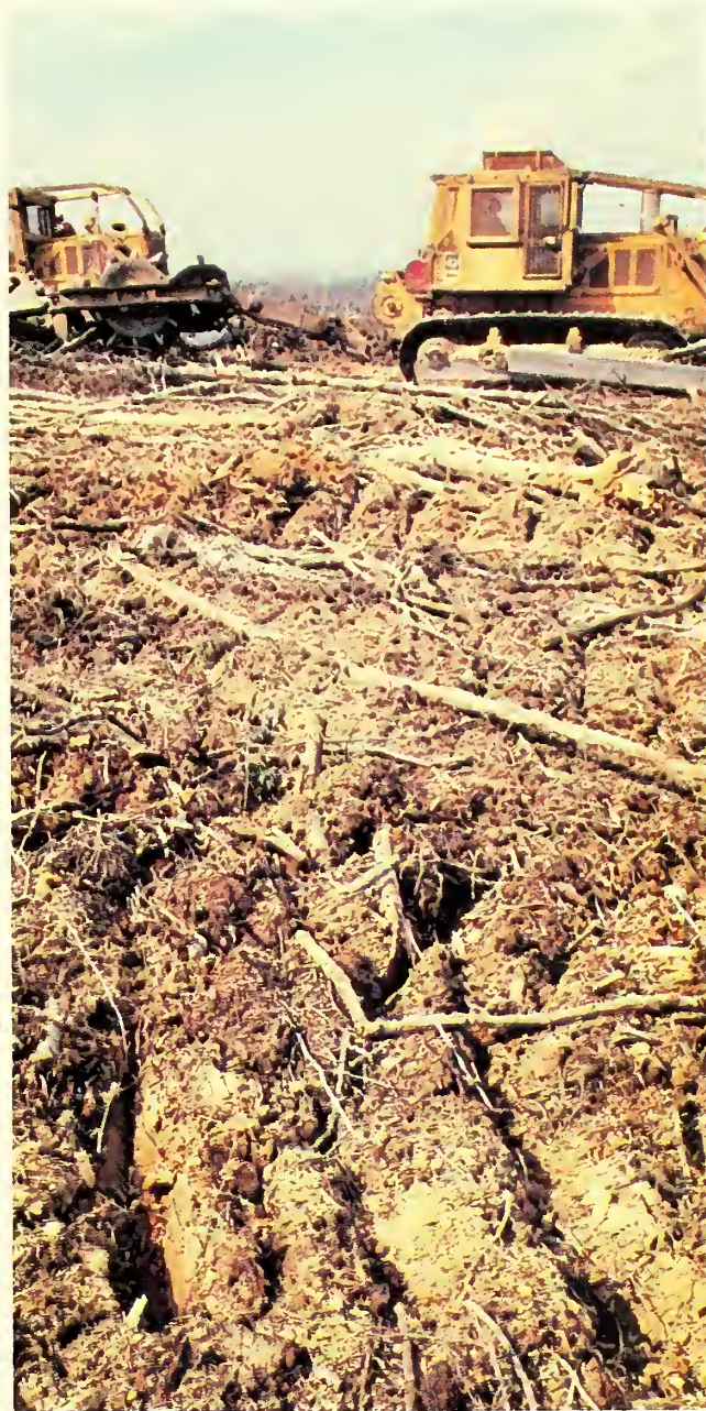
Figure 22.—Chopper slits trapping most of the erosion, with a rating of 0.1.
